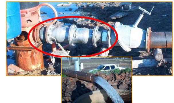
Installed on Irrigation system
