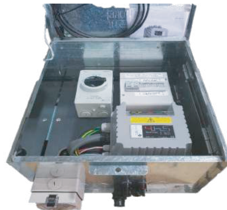
ENC350 With AC/DC Switchgear
